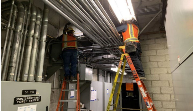
System Installation at Wilshire/Western
