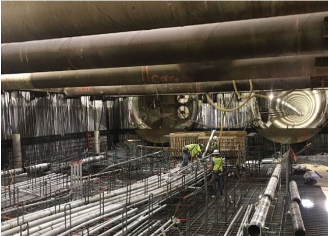
Embedded conduits at WRS (West Hammerhead)
