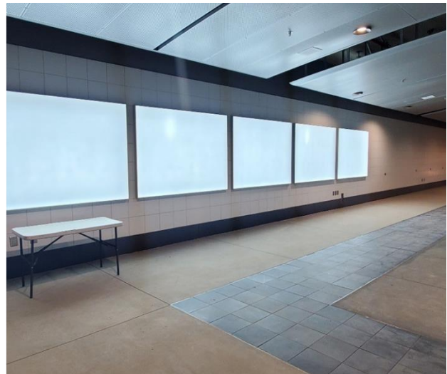
Installation and wiring of photographic light boxes at Concourse Level at Grand Av Arts/Bunker Hill Station Upper Plaza
