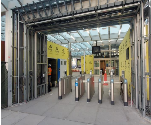
Installation of glass exit door at Little Tokyo/Arts District Station north Plaza
