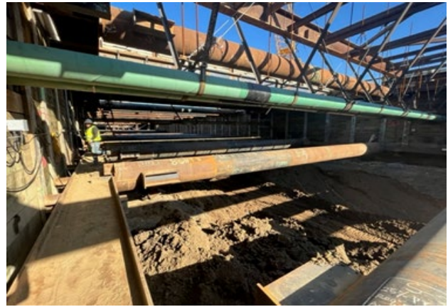
Westwood/VA Station Installation of Level #2 Struts & Strain gauges; Utility Supports Shown Above
