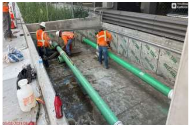
SD drain piping for Broad Museum planter
