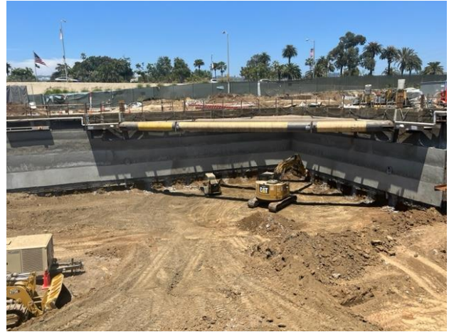
Installation of Level 2 Tiebacks & Level 3 Shotcrete at the Westwood VA Station Entrance
