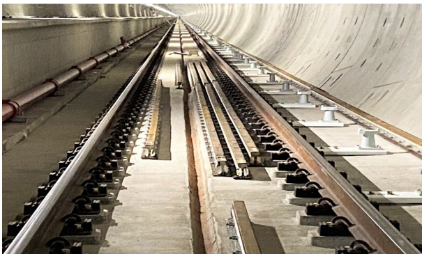
Reach 1 BL Tunnel Contact Rail
