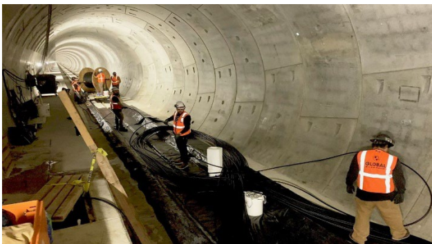
Reach 1 (BR) Communications Installation
