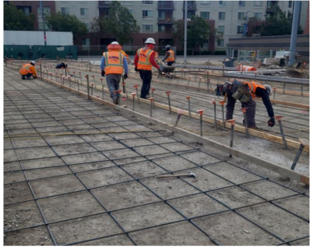
Formwork for the Little Tokyo/ Arts District Station Plaza Level architectural concrete
