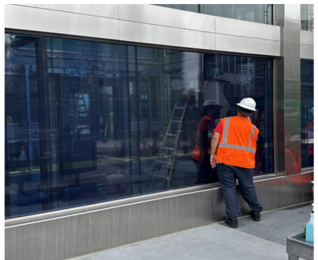
Vinyl artwork along elevator tower glass panels at the Grand Av Arts/Bunker Hill Station
