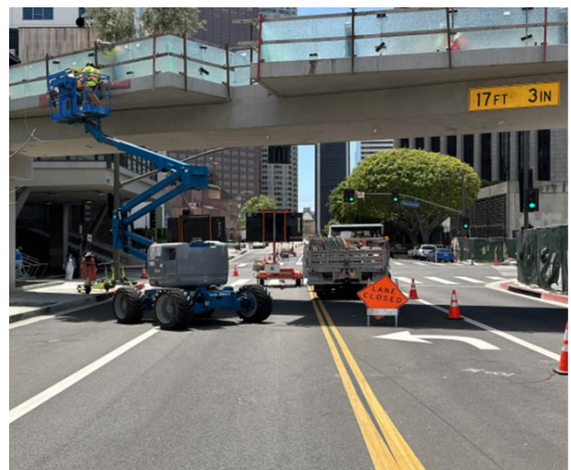
Epoxy pour to set glazed panels along Ped Bridge connected to Grand Av Arts/Bunker Hill Station
