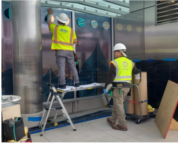
Graffiti shield film installation on art glass at Little Tokyo/ Arts District Station Plaza Level
