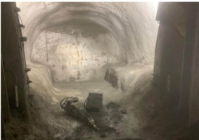
Completed Excavation and Lining for TH and center Bench Up to BL Segments
