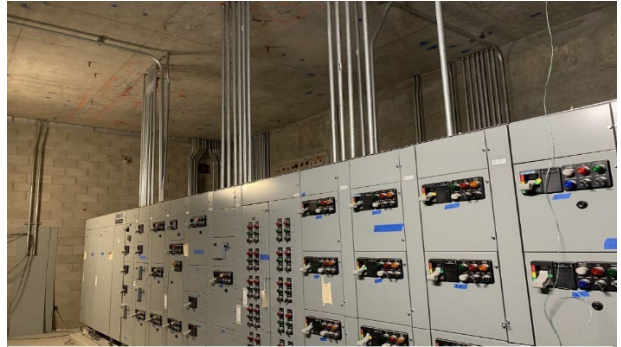
Motor Control Centers (MCCs) at Wilshire/La Brea Station
