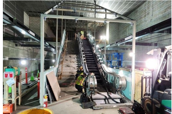
Wilshire/Fairfax Station Escalator Assembly (Platform to Concourse)
