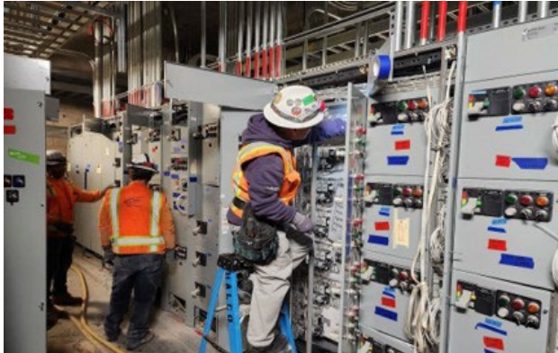
Wilshire/La Brea Station Motor Control Center (MCC) Cable Terminating (Aux Power Room 303)
