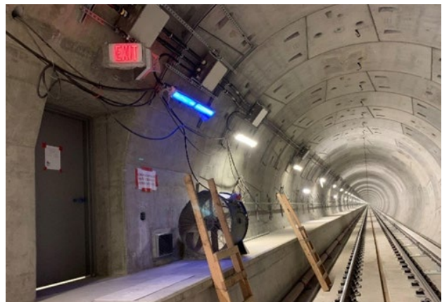
Reach 1 Tunnel Lighting Energization
