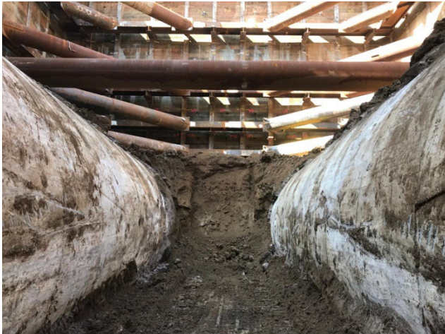
Westwood/VA Station: Excavation at Level 4 to 5 Between the BR & BL Tunnels at the West Hammerhead
