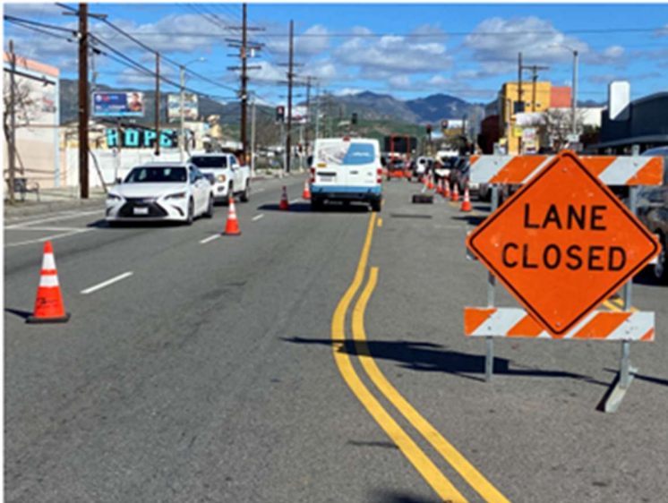
Traffic Control for Operation to mark Phase II Hazardous Materials Boring Location and check for the Underground Utility Conflict
