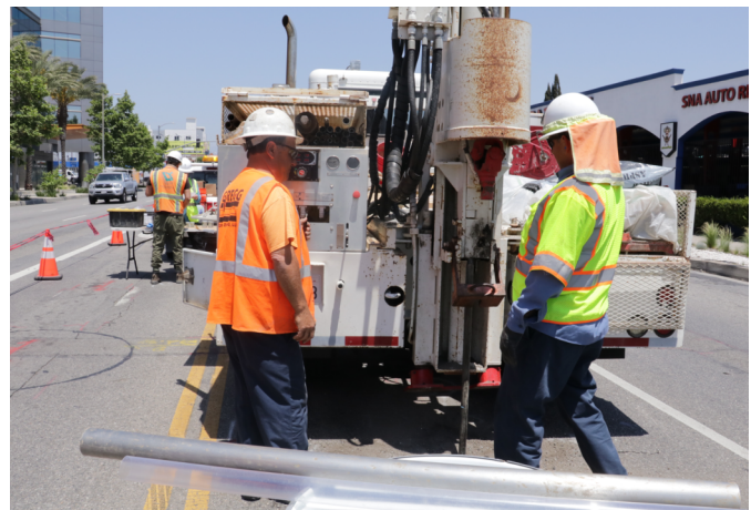
Gregg Drilling: taking core sample for soil analysis at Covello and N. Van Nuys Blvd.
