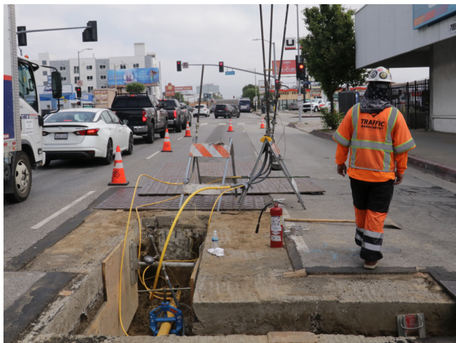
Southern California Gas Company: Relocation of gas line at 7654 N. Van Nuys Blvd – Testing of the new gas line
