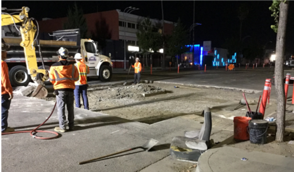
WA Rasic: Breaking and removing asphalt to replace with new at Vault 6900
