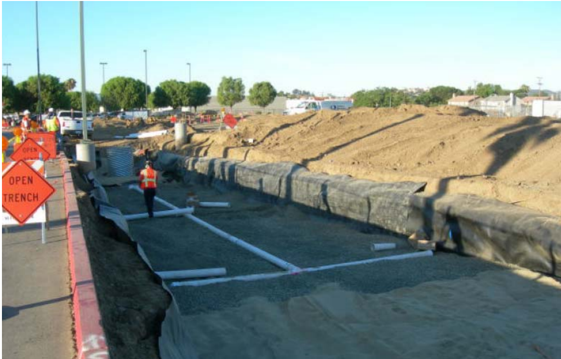
C0941 North Parking Lot Sully-Miller Contracting Co. constructing bioinfiltration facility for water quality mitigation measures.
