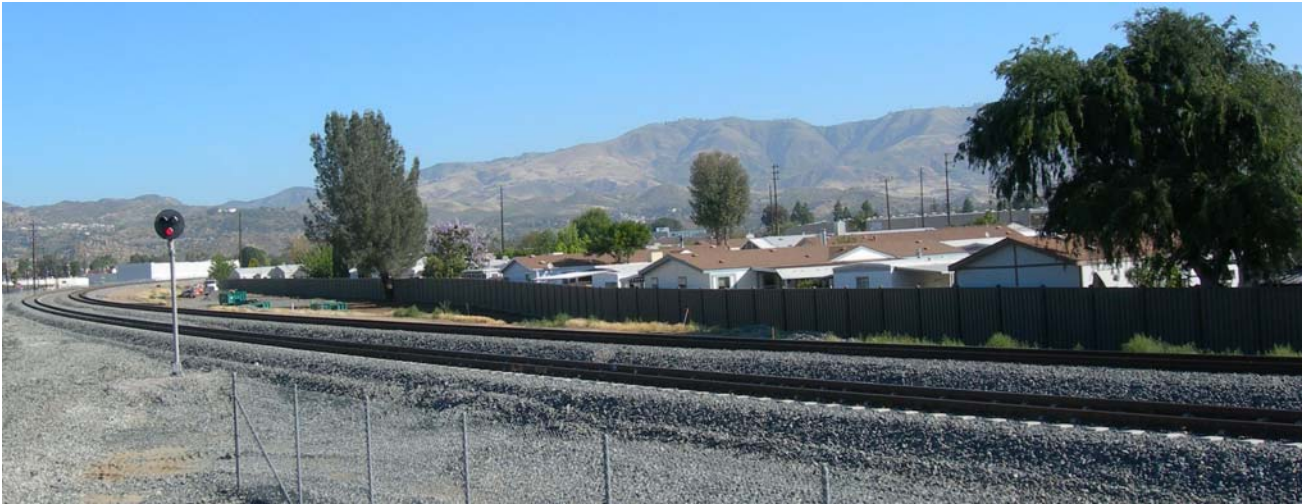
Completed construction of new privacy fence at Chatsworth Mobil Home Park in advance of Lassen Bridge construction.
