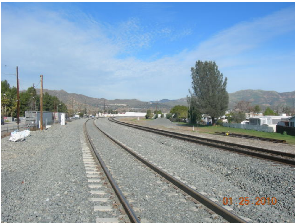
SCRRRA replaced 3,300' of tracks between Lassen Street and Brown's Creek in advance of start of construction.
