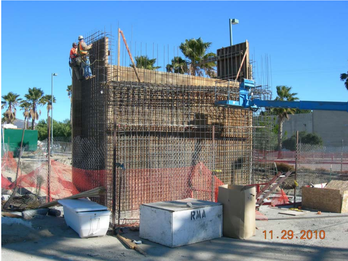
C0943 Design Build Contractor installing wall reinforcing steel for Lassen Bridge abutment # 4.
