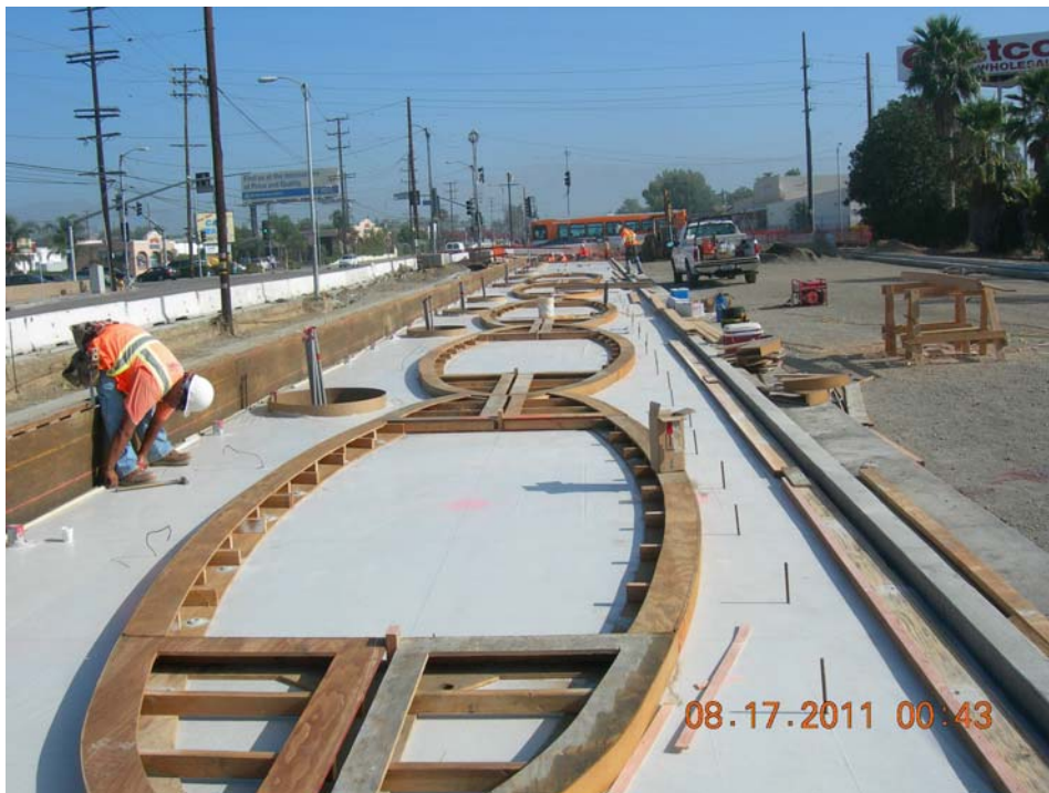
C0943 Design Build Contractor working on formwork for Roscoe Station (south platform).
