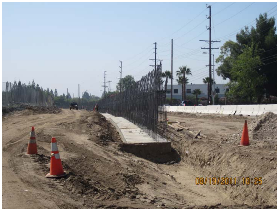
C0943 Design Build Contractor working on retaining wall at pinch point (Canoga Avenue).
