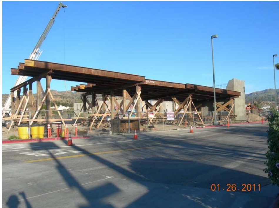
C0943 Design Build Contractor installing falsework between Abutment # 4 and bent # 3 for the Lassen bridge.
