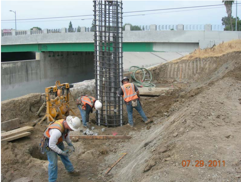
C0943 Design Build Contractor placing CIDH piles 1 & 3 at the Los Angeles River Bridge.
