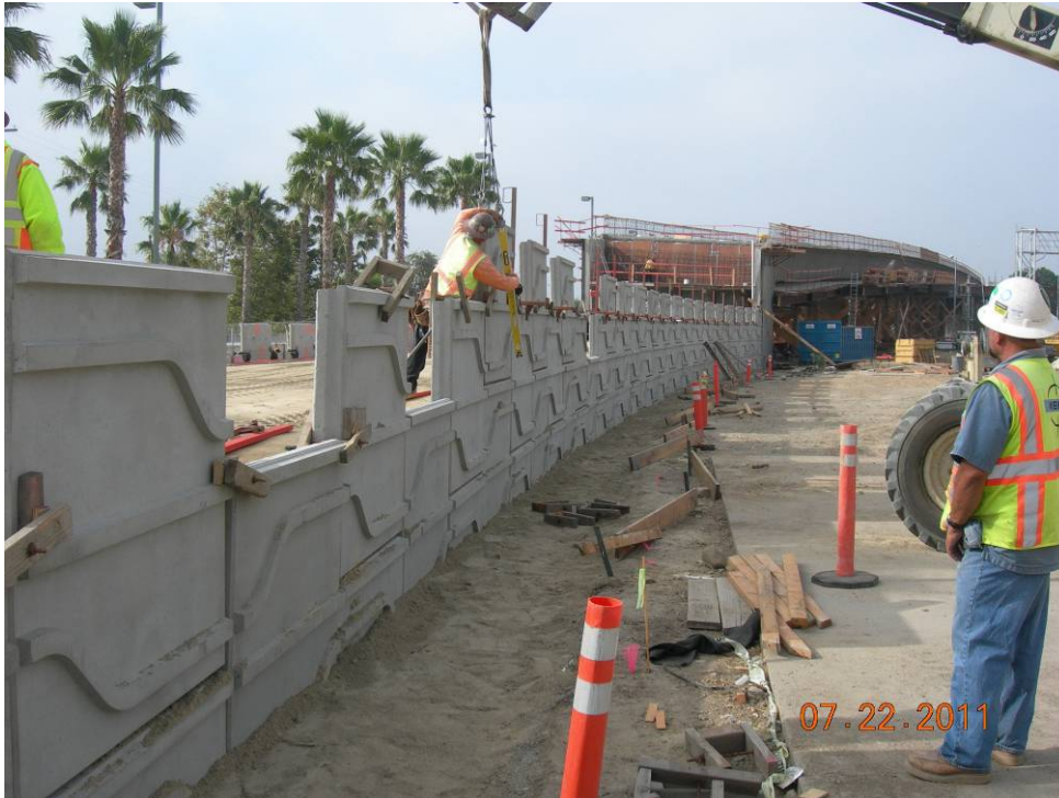
C0943 Design Build Contractor placing mechanical stabilized earth walls leading from Lassen Bridge into Chatsworth Station.
