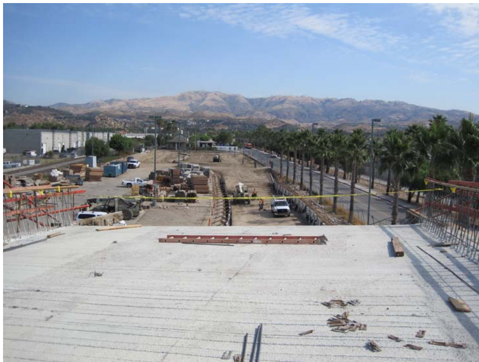
View from on top of placed deck for Lassen Bridge looking north to Chatsworth Station.
