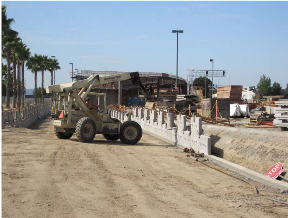
C0943 Design Build Contractor works on mechanical stabilized earth wall leading from Lassen Bridge into Chatsworth Station .
