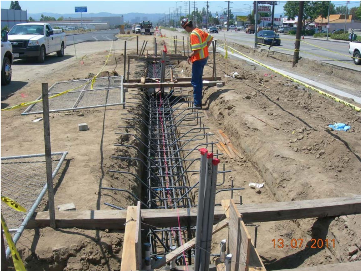
C0943 Design Build Contractor works on piles and grade beams for Roscoe Station platform.
