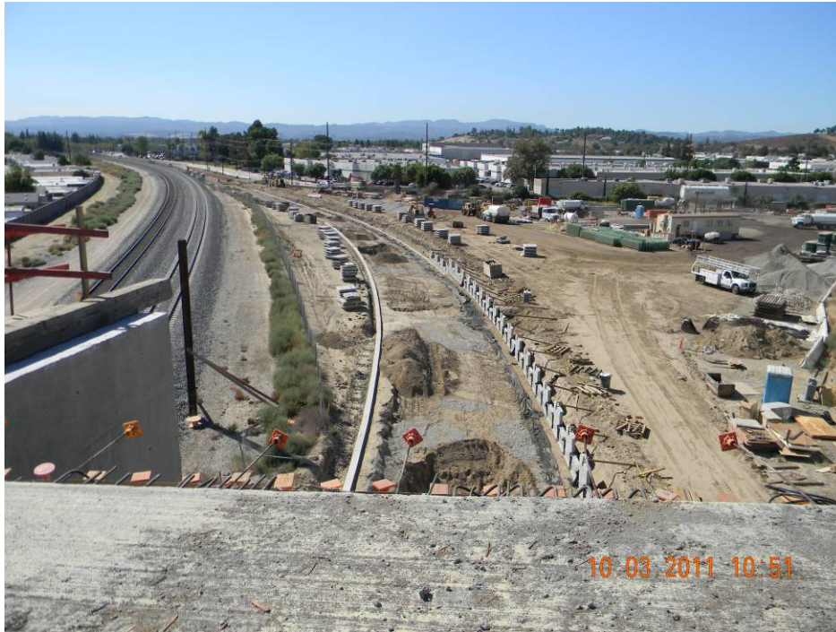
C0943 Design Build Contractor working on mechanical stabilized earth walls 1 and 2 at Lassen Bridge.
