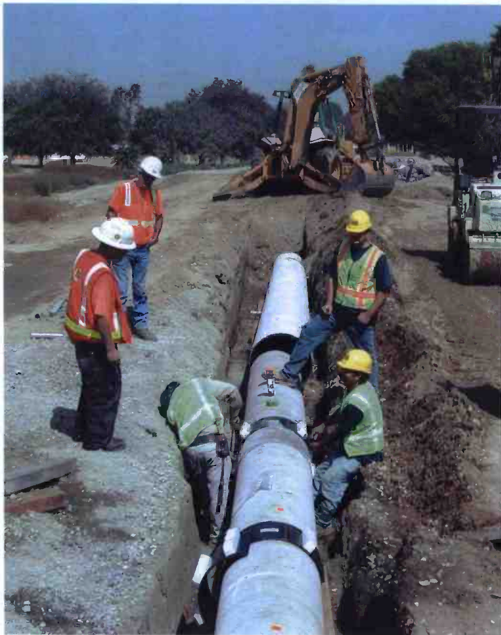
Contract C0676 Los Angeles River Bridge Contractor installing LADWP Recycled Water Pipeline adjacent to Bridge.
