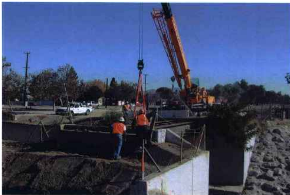
Contract C0675 Design/Build – Crane operation in progress at Bull Creek Bridge – one of two new bridges to be built by Contractor.
