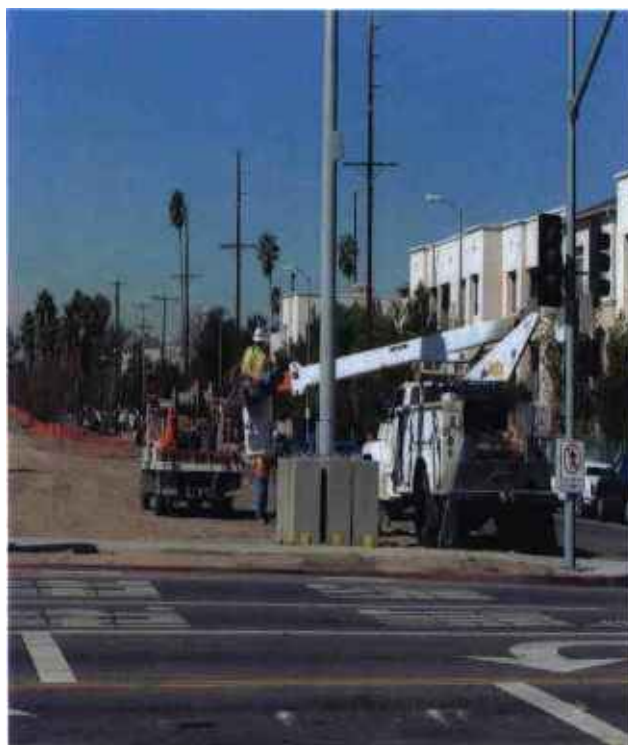
Contract C0675 Design/Build Contractor completed Temporary CCTV pole and foundation installation at Coldwater Canyon.
