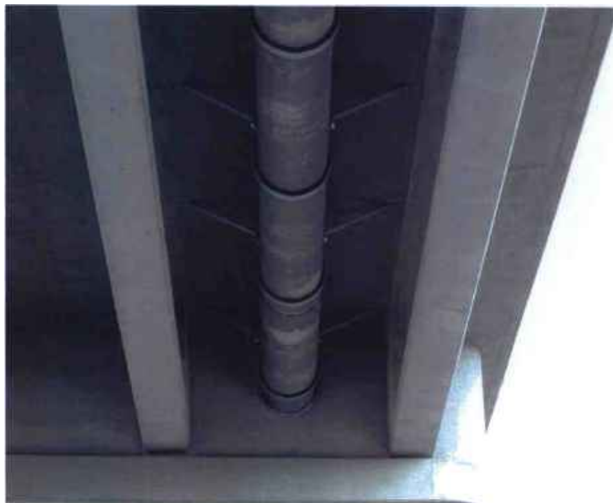
Contract C0676 Los Angeles River Bridge Contractor completed installation of LADWP Recycled Water Pipeline under Bridge.
