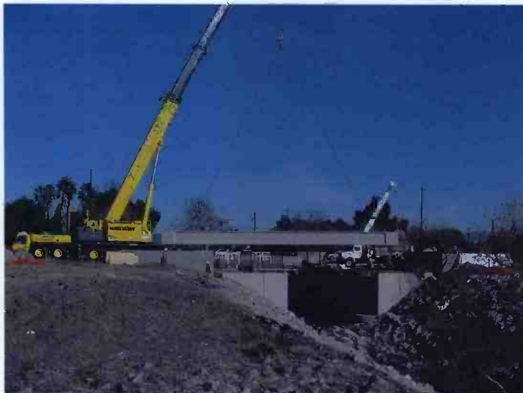
Contract C0675 Design/Build girder installation at Bull Creek Bridge – one of two new bridges to be built by Contractor.
