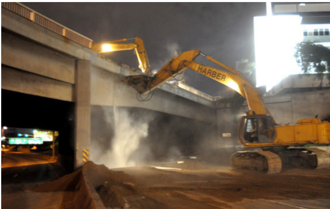
The hoe ram at work on the Flower Street bridge over the 110 Freeway downtown
