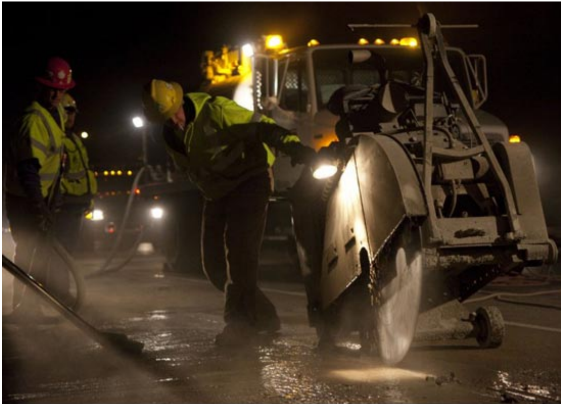
Night work on the freeway in March, south of Getty Center Drive/Metro photo
