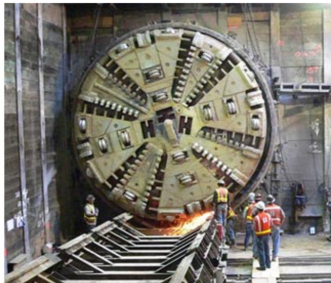
“Closed face” Earth Pressure Balance tunnel boring machines were first used by Metro in the Gold Line Eastside Extension
