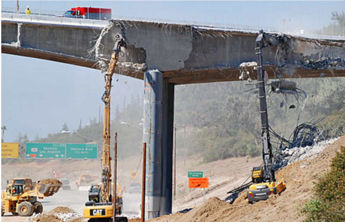
By late afternoon, crews had made substantial progress in tearing down the Mulholland Bridge's south span.
