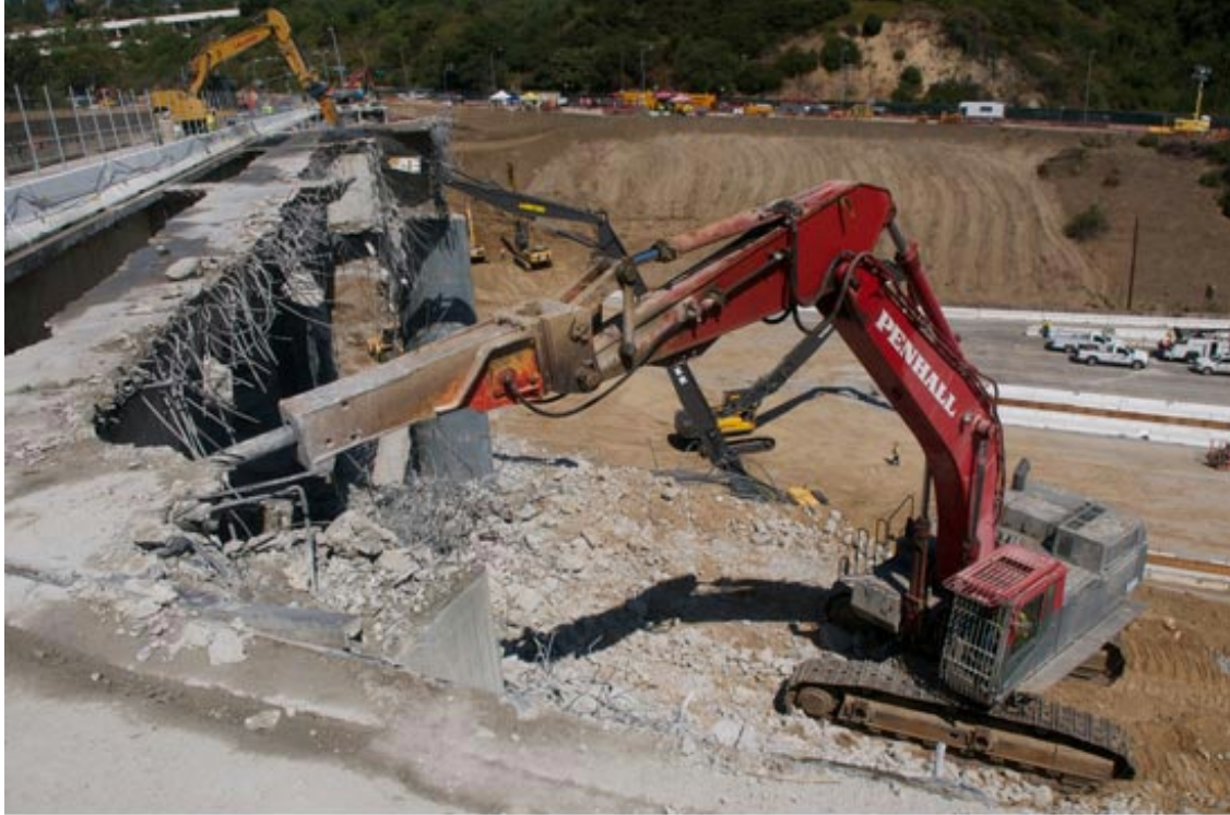
The Mulholland Bridge was partially demolished during “Carmageddon” in July. Metro photo by Gary Leonard
