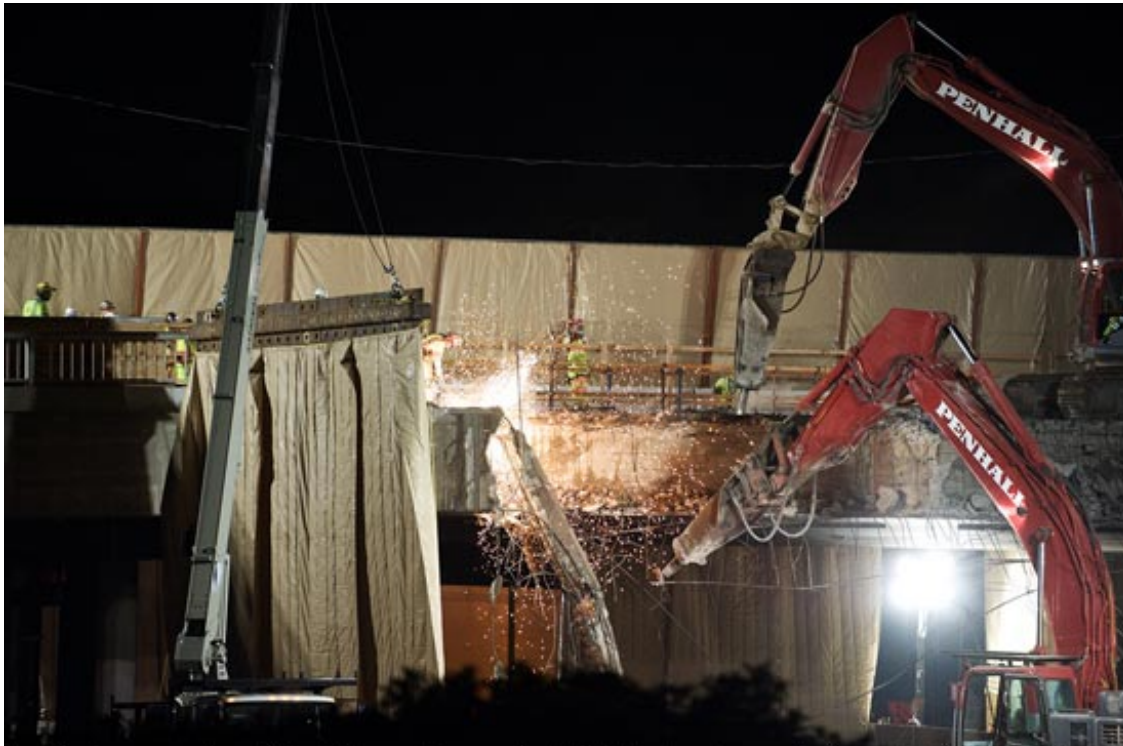
Duet for hoe rams: Two of the giant machines go about their business in a work site swathed in sound blankets.
