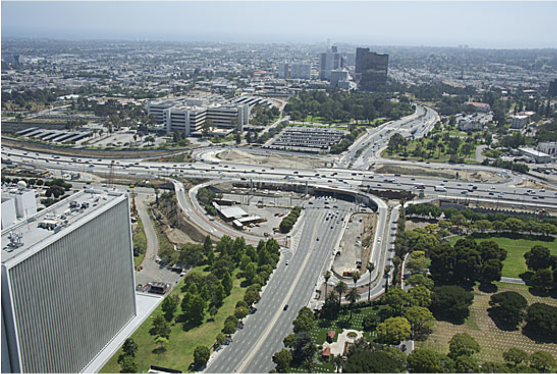
The Wilshire ramps will be undergoing a year-long reconstruction. Photo/Gary Leonard for Metro
