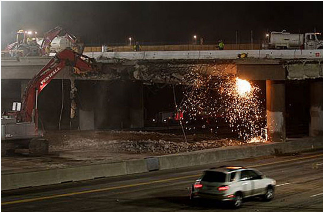
The north side of the Skirball Bridge came down in 2010. Now it's time to demolish the south side.
