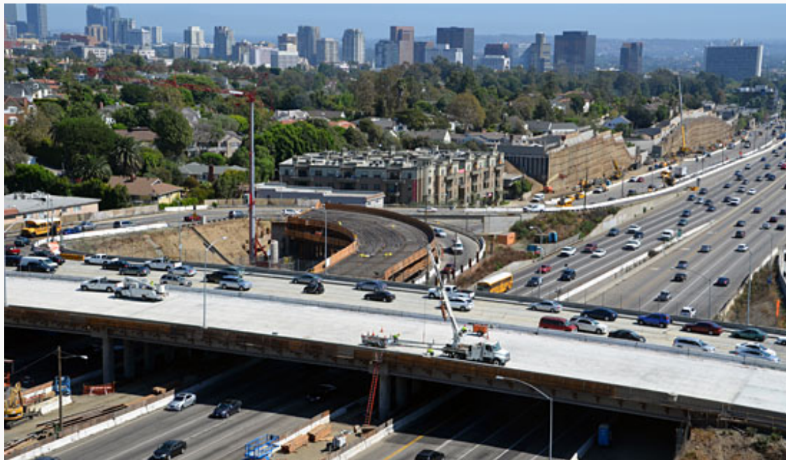
After more than two years of work, the Sunset Bridge is back in action starting Monday. Photo/Metro
