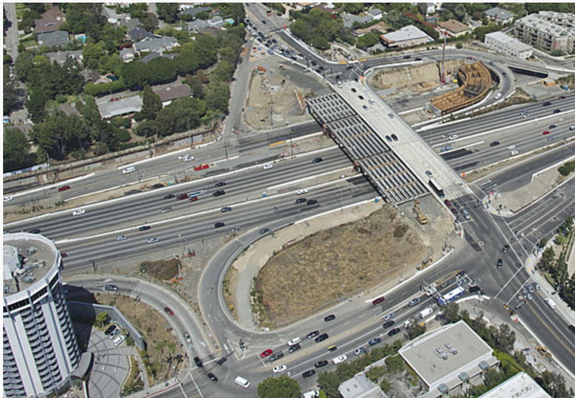
Sepulveda Boulevard, which runs along the 405, is closing between Montana and Church every night this week. Photo/Metro
