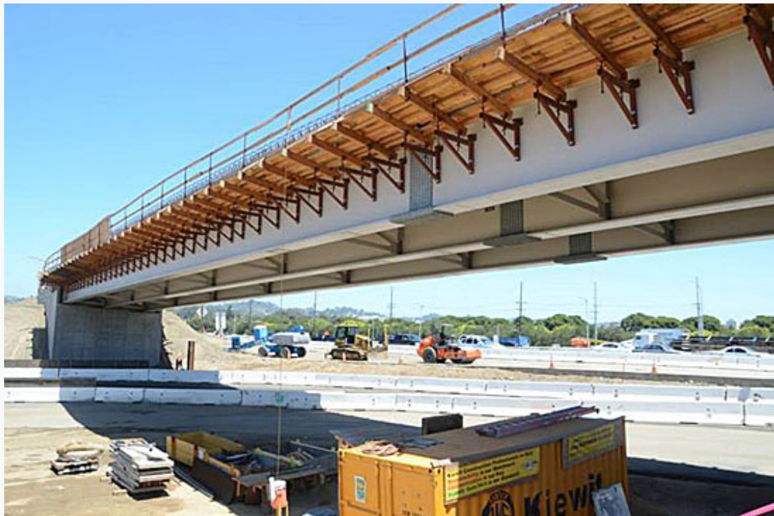
This flyover ramp, photographed in May, is part of the Wilshire segment nearing completion. Photo/Metro
