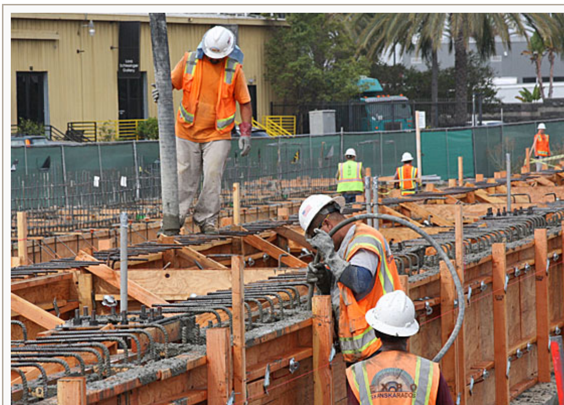
Workers construct the Expo Line platform at 26th Street in Santa Monica.
