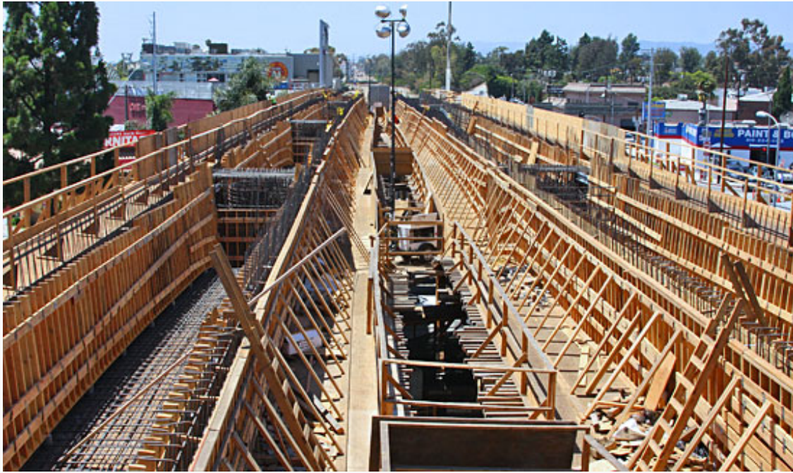
The Venice Boulevard Bridge, under construction last week. Photo/Dwight Sturtevant for Expo and Metro
