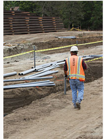
On the job at the future Westwood Station. Photo/Dwight Sturtevant for Expo and Metro
