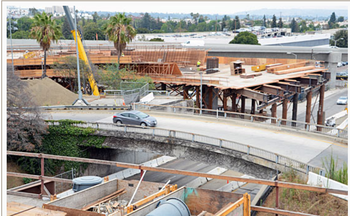
The current northbound on-ramp from eastbound Wilshire, shown at center, will be demolished. Photo/Metro
