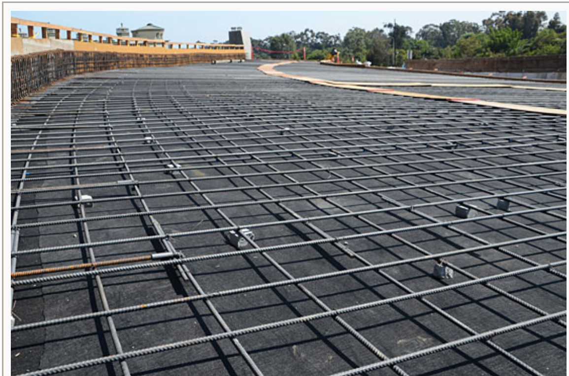
A new Sunset off-ramp takes shape in advance of a lengthy closure starting next month. Photo/Metro
