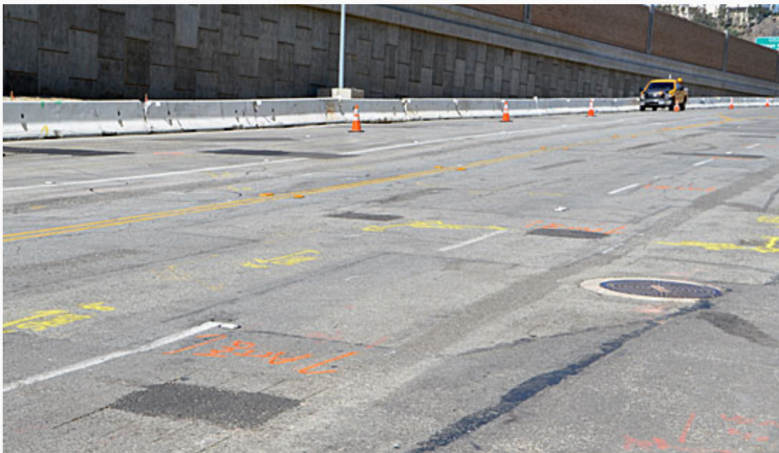
Reconstruction and paving will smooth a patchwork of surfaces on Sepulveda. Photo/Metro
