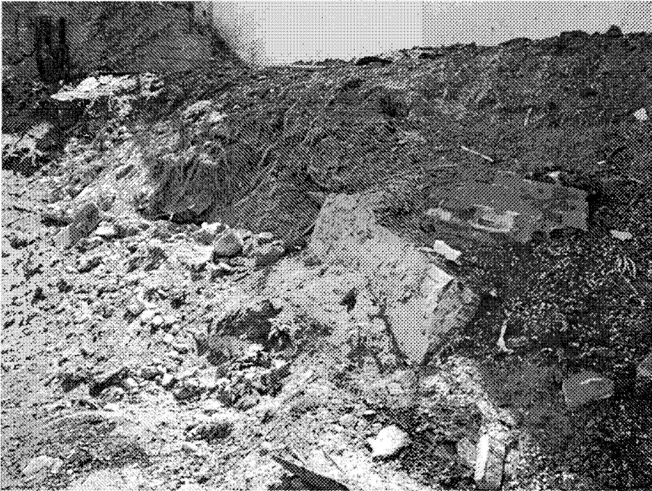
Figure 17. Exposed brick conduit near project area west section
