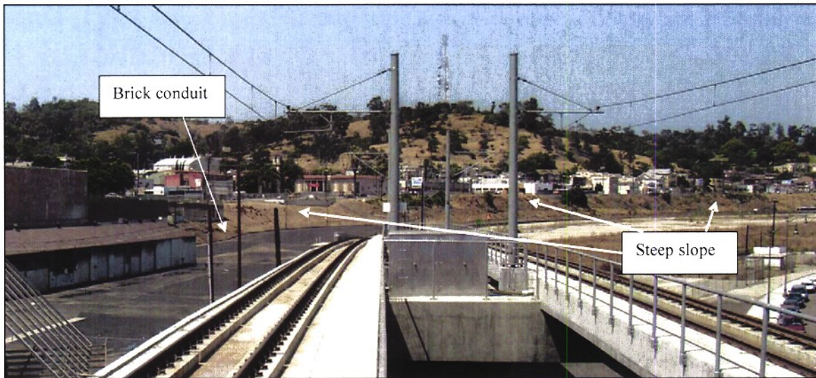
Figure 2.5. Location of exposed brick conduit (2000 segment) on private property northeast of Gold Line platform
