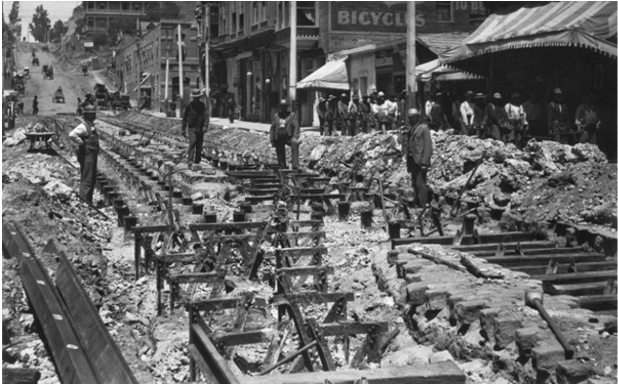
Workers dig up abandoned cable car railway tracks on Second Street. Courtesy of the Metro Transportation Library and Archive.
