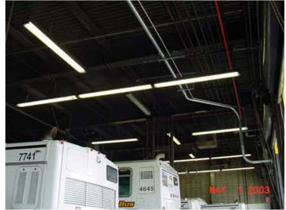
Existing Repair Bay Lighting
