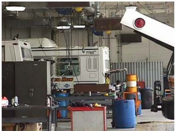
Low Ceiling in Maintenance Bays
