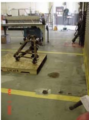
Shop Flooring Damage
