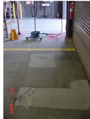
Shop Flooring Patch Failure
